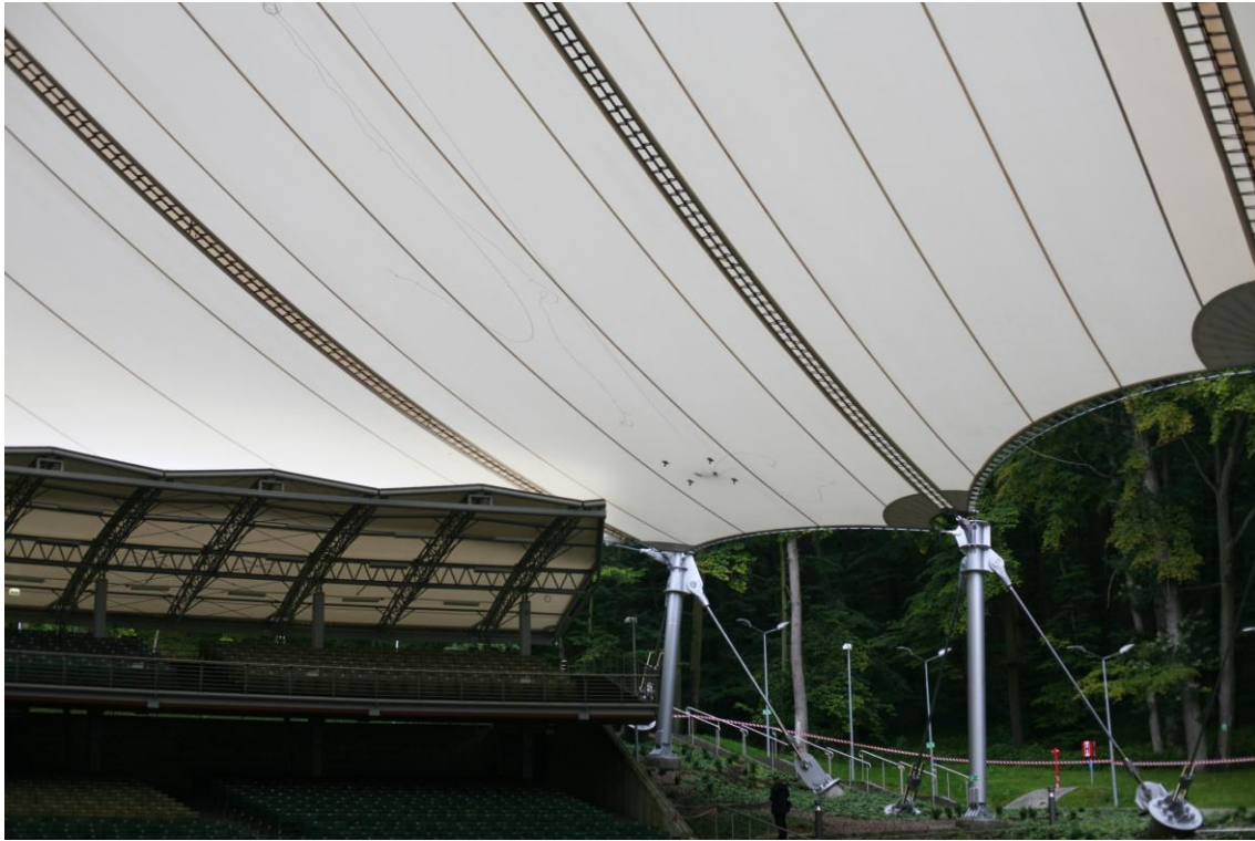
Fig. 5. View onto the Opera covering with GMP104 prisms installed on the membrane.
