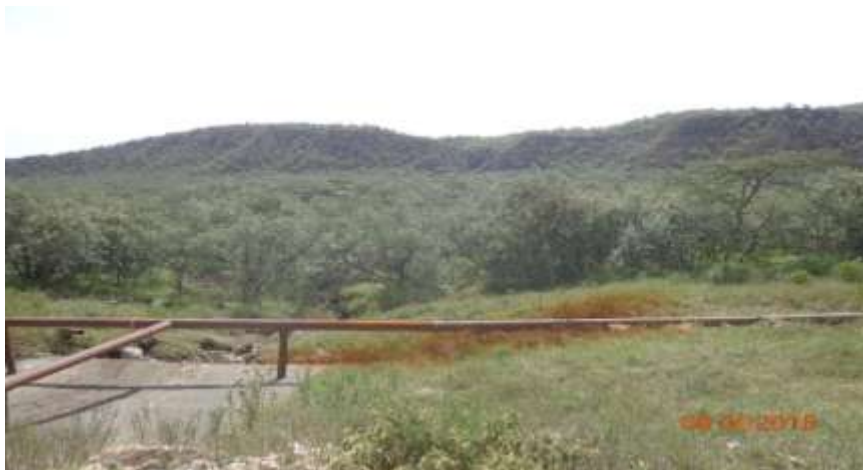
Plate 1: Leaking steam gathering system
