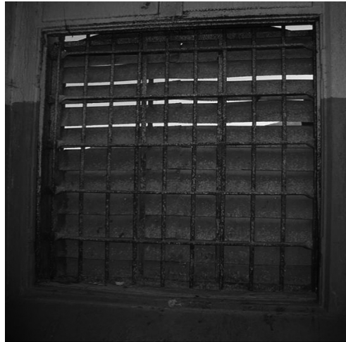
Figure 3. “Security blinds” impeding proper ventilation and sunlight from coming into the cell.
