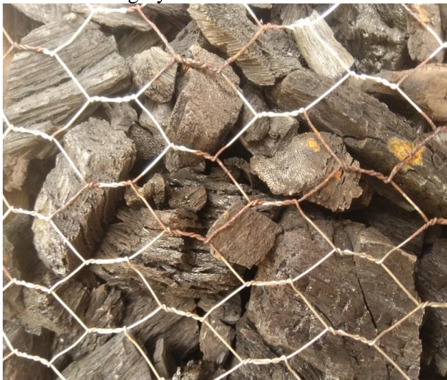
Fig. 8 Rusting and mineral deposition effect
