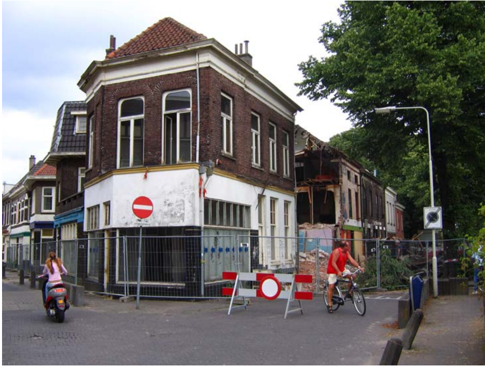
Figure 1. Property of Volkshuisvesting Arnhem - the Arnhem fashion district Klarendal: before the renovation.
