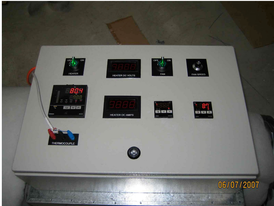
Figure 19 Close-up view of thermal test rig heater/fan assembly. Display unit at centre/left is heater PID controller. To the right are displays showing DC voltage and current of heater.
