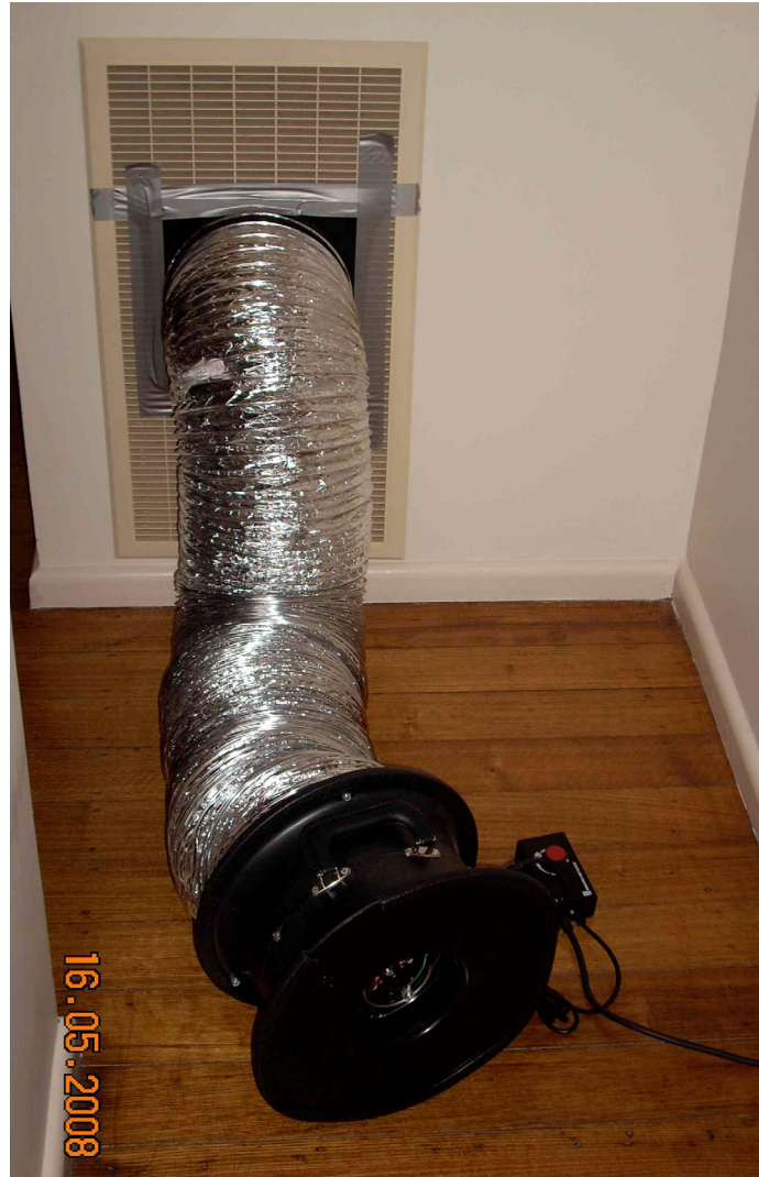
Figure 10 Duct Blaster fan connected to return air grille before grille is completely sealed.
