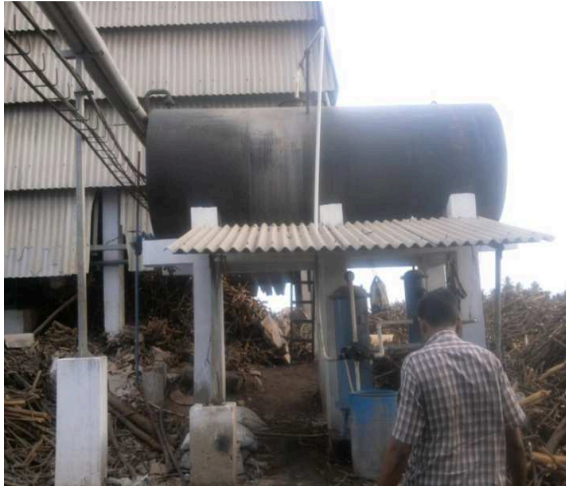
Fig. 2. Feed water tank
