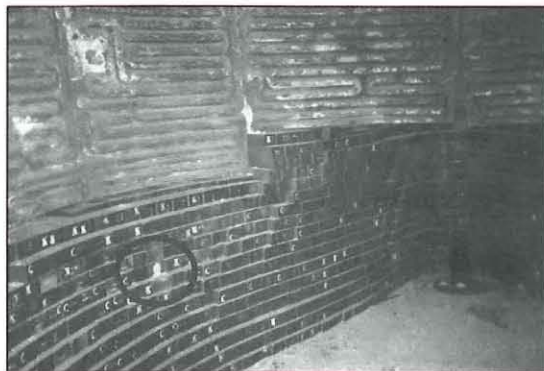
● Figure 2 Inside view of EAF showing lance position
