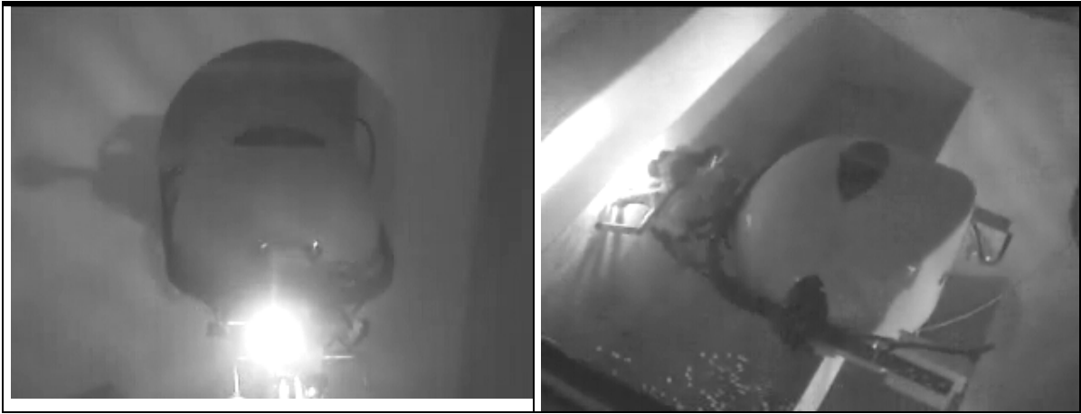
Fig.19: Photograph of ROTIS passing through a horizontal manhole Fig.20: Photograph of the docked ROTIS while perform visual inspection and wall thickness measurements.
