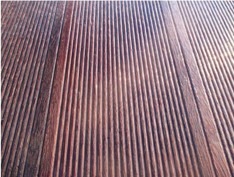
Figure 4: Bangkirai test deck, originally with 5 mm gaps totally closed up after being exterior exposed.
