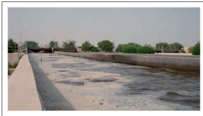
Figure 2. An oxidation ditch consists of a long channel where sewage water is injected with oxygen and bacteria to decompose the waste for around 14 hours.
