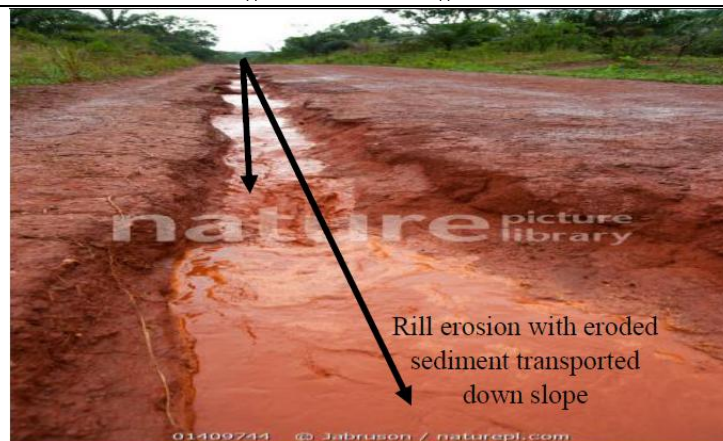
Fig. 4. A rural lateritic road damaged by erosion in the Central African Republic. Accessible at https://www.naturepl.com/stock-photo-erosion-of-murram-road-after-rainstorm-in-wet-season-boukoko-village-image01409744.html
