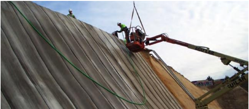
Figure 13: Concrete Canvas applied to slope protection (Image: Courtesy of Concrete Canvas Ltd)
