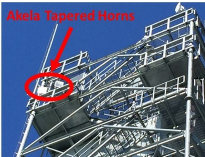
Figure 9. Akela tapered radar horns (1 transmit, 1 receive) mounted to the STS tower, 110' above ground (outlined in red).
