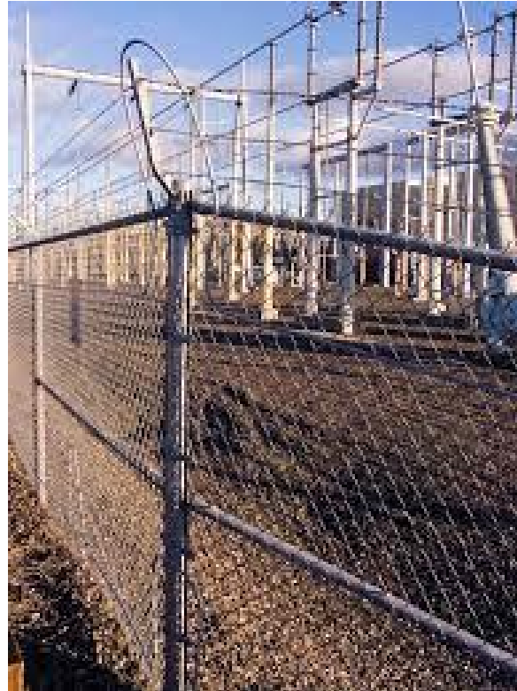
Fig. 1: A fibre optic perimeter security mounted in a barb-wired fence to protect power station
