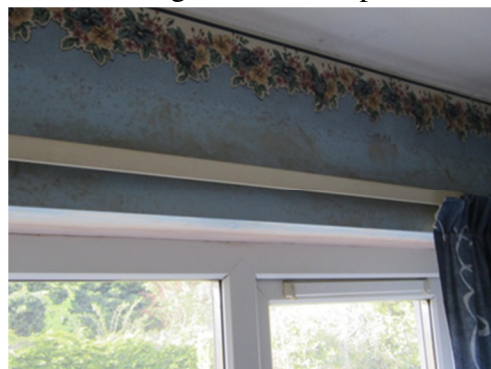
Figure 5: Staining on external wall due to condensation
