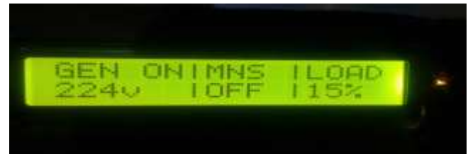
Figure 13. Screen display when generator is ON and mains is off
