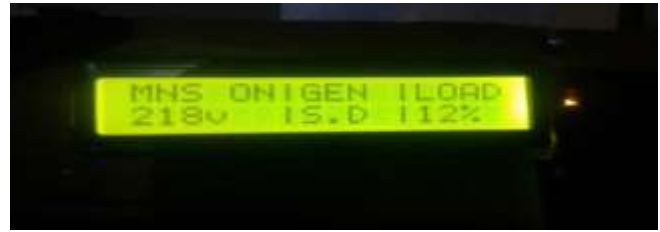
Figure 10. Screen display upon generator shutdown
