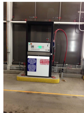
Figure 3 Compressed Natural Gas station inside maintenance facility.
