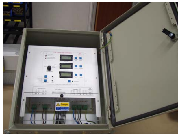
Figure 9: Control box layout
