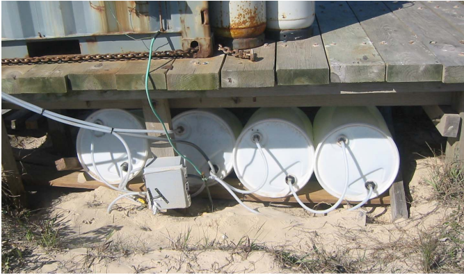
Figure 3. Water cooling reservoir installed at Matagorda Island site.
