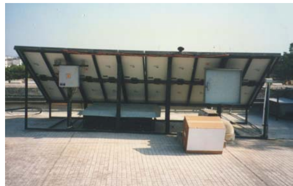
Figure 2: The first solar PV stand-alone system to be tested in Malta (1993-1995). A battery bank was placed underneath the modules and a battery charge control unit is seen to the left. Monitoring equipment was placed in the box to the right.
