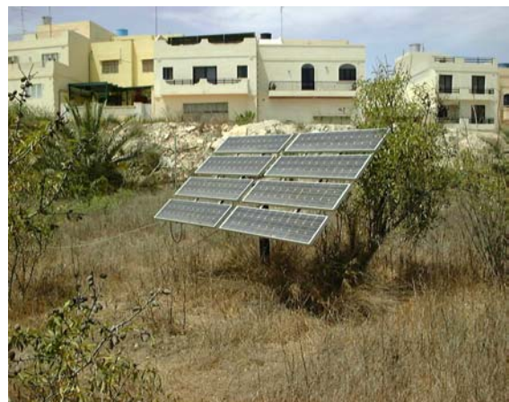
Figure 1: A solar photovoltaic water pumping system, installed at the Institute for Energy Technology since 1985.
