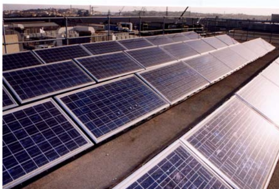
Figure 6: Malta’s first and currently largest grid-tied solar PV system in an industrial area.
