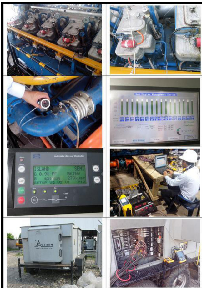
Figure 3. Details of the base instrumentation used during the test of generator sets.
