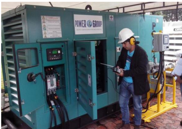
Figure 4. Generator set based on BIFUEL-CUMMINS 6CTAA8.3-G1
