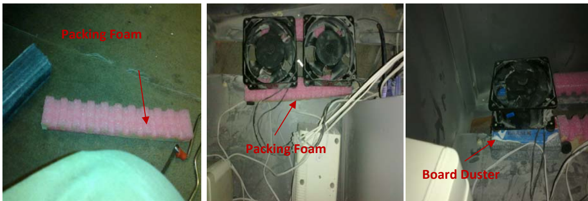
Figure 12 - Fan placed on Packing Foam (center) and blackboard duster (right)
