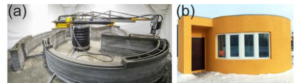
Figure 9. On-site’ 3D printed house by Apis Core (a): Construction using a ‘mobile’ 3D concrete printer, (b): House exterior [19]
