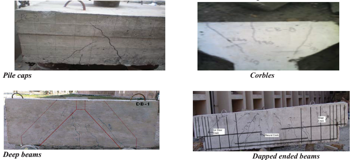
Fig.6 Typical failure modes of deep pile caps, corbelsl, deep beams and dapped ended beams.
