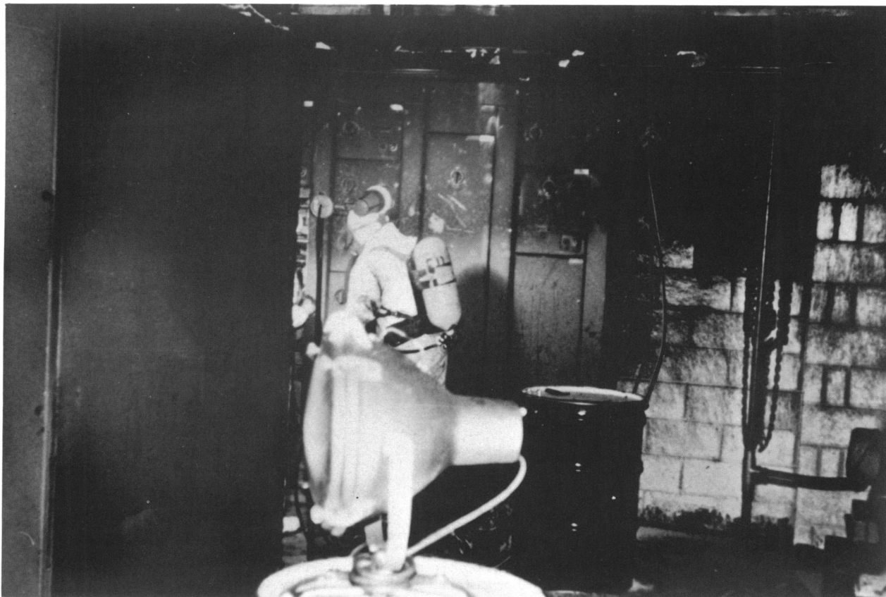
FIGURE 4. A worker wearing full air pack, self-contained breathing apparatus (SCUBA) and full face and body protection is shown working in the transformer room.
