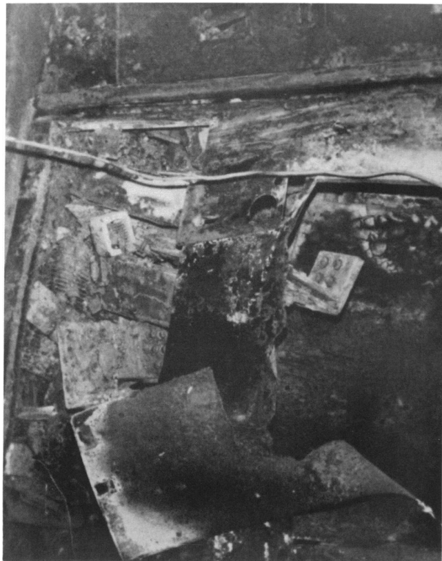
FIGURE 9. Intense heat at the electrical panel produced this damage. Metal panels are destroyed or bent by the heat of the electrical arcing.
