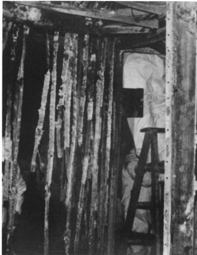
FIGURE 10. The intense heat burned the insulation from these wire cables. This implies other chemicals such as vinyl chloride may have been involved in the initial worker exposure, especially that of firefighters, police and supervisory workers, as well as photographers and other representatives of the press.
