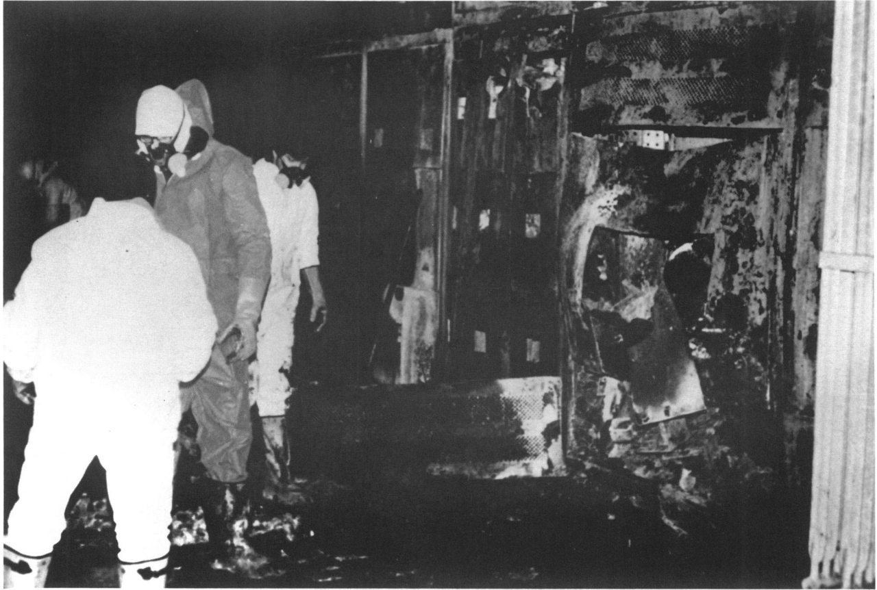
FIGURE 3. This photograph shows the damaged, soot-covered, electrical panel and several workers wearing different sorts of protective clothing over their street clothing. Respirators with cartridges filtering air and particulates are apparently being worn by these workers but full facial protective masks or oxygen breathing apparatus are not being used. These photographs were taken in February 1981.
