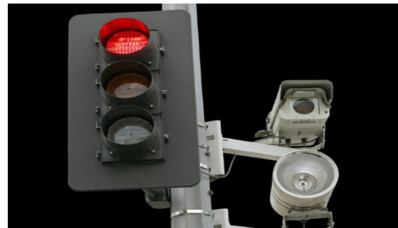
Figure 2: Cameras installed on red light.
