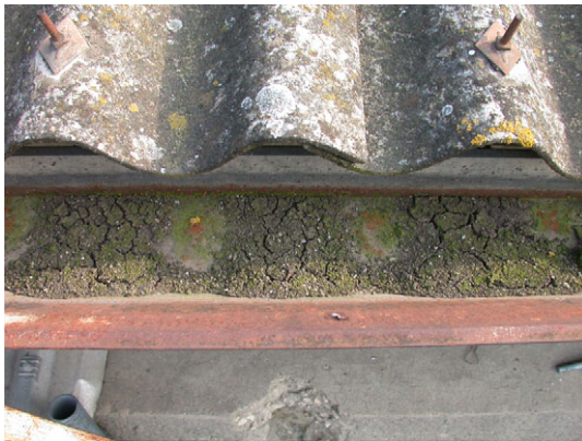
Fig. 2. Friable material in the gutter.
