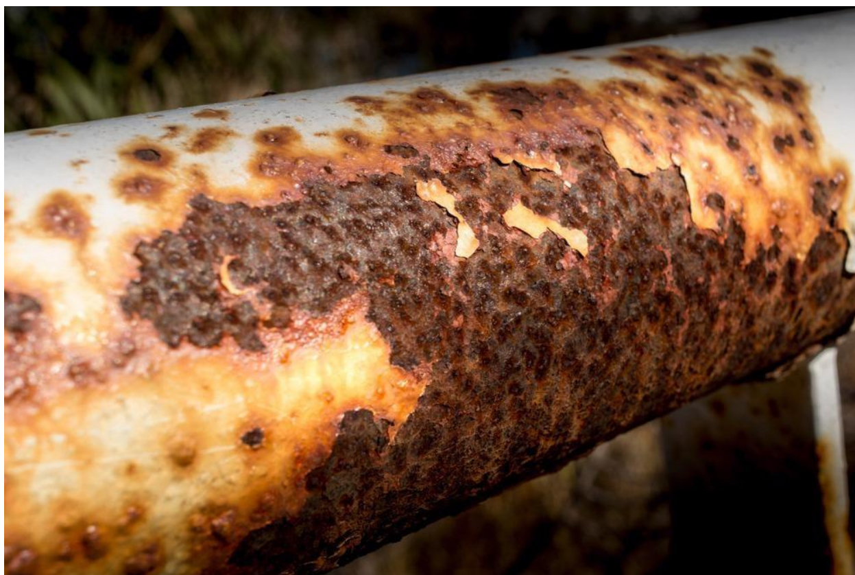
Figure 1. Corrosion of metal.
