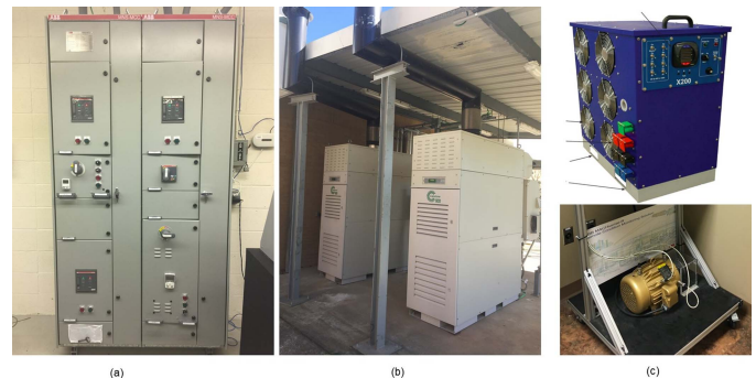
Figure 2. Components of McNeese MG. (a) MG control center (b) CHP generators and (c) resistive and rotating load with sensors attached to it
