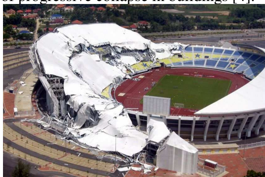
Fig. 1: Picture of the collapse of the Sultan Mizan Zainal Abidin Stadium , Malaysia [5]
