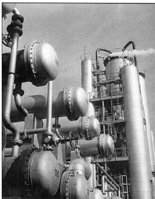
Fig. 17. Atmospheric-vacuum distillation 3 of crude oil in Slovnaft with capacity of 1.3 mil ton/year after intensification.
