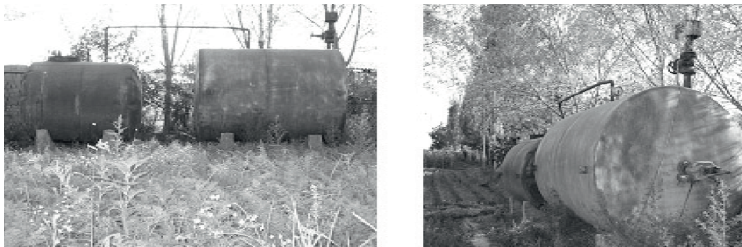
Fig. 3: Biogas digester installed in Rudaki district of Tajikistan.
