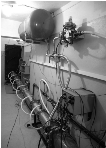
FIGURE 1. Pulsed detonation combustor operating on natural gas and air. The open end (far end) is immersed into a furnace.
