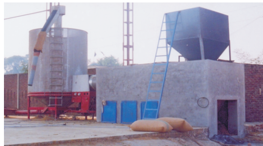
Figure 3. A typical view of the rice husk-fired cross-flow dryer
