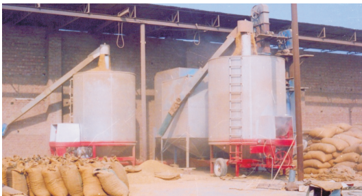
Figure 2. A typical view of the gas-fired cross-flow rice dryer
