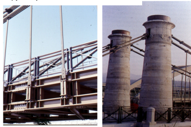
Figs. 6 and 7: Details of the mesh of the Vierendeel type girder and of the masonry piers
