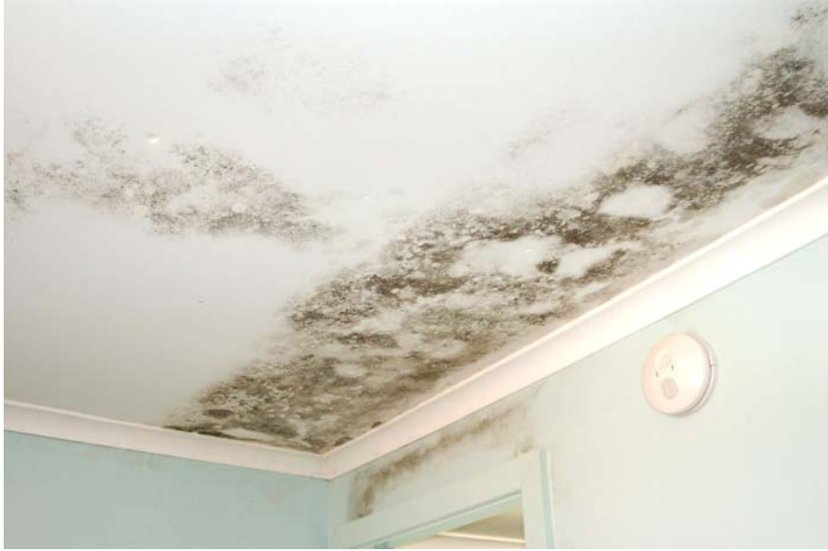
Figure 1 Grade 4 Mould contamination on ceilings
