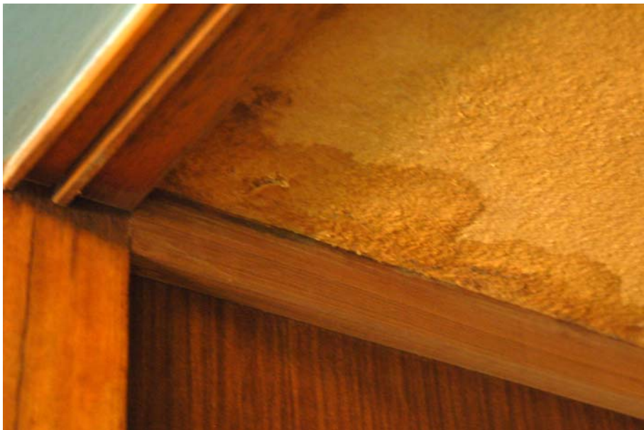
Figure 2 Water staining insides of built in wardrobes
