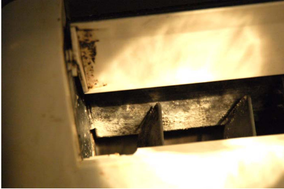
Figure 3 Mould Contaminated air conditioning fins
