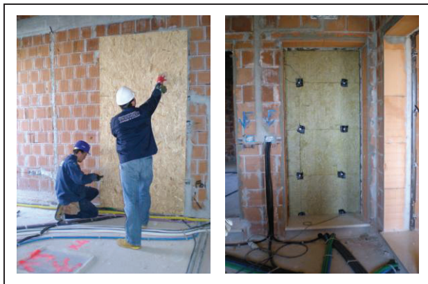
Figure 4. Example of installation of a temporary door. The sound absorbing side of the panel is placed outside the measuring room.
