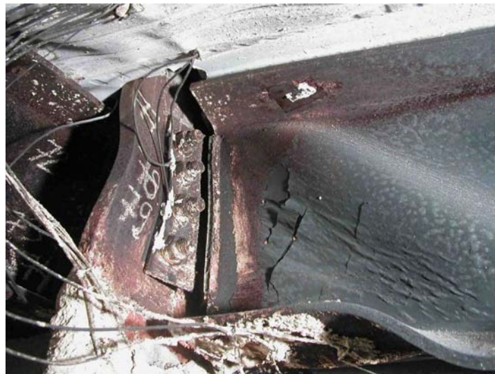
Figure 1: Fracture of the end-plate
